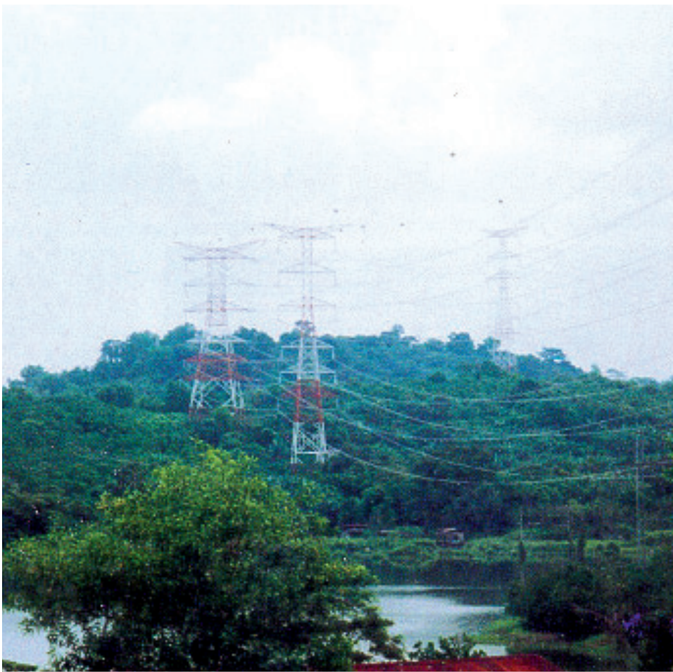
A view of river crossing towers in Malaysia
